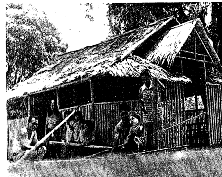
Elder E. Gulfan and Rev. E. Ferraren are shown working on the new bamboo church in Cebu City, the Philippines. The women also contribute to the new building. Mrs. Corazon Gulfan is shown preparing a beam.
