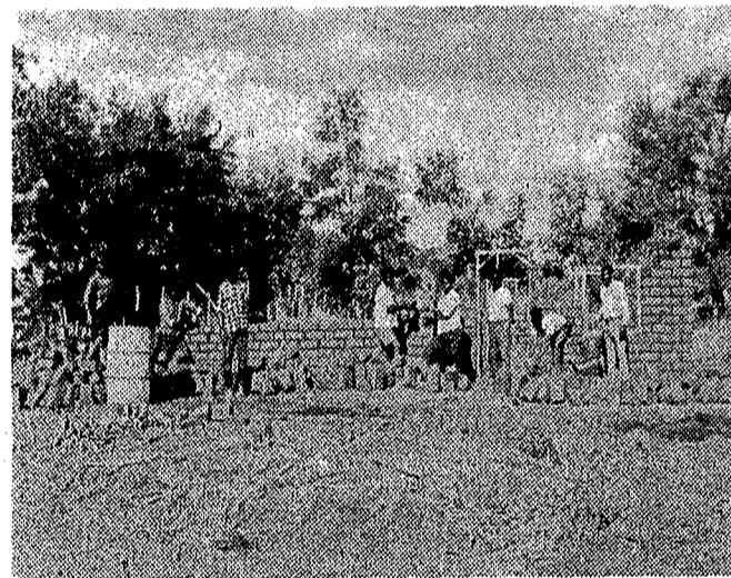
The house is now about to be complete. It has seven rooms, including an office that will be used by Pastor Mataka to translate the Sabbath School lessons - The Helping Hand , for Malawi. The roof is made of grass. The people are now concerned with the grass roof and are thinking on the means to improve the roof to a metal one.
