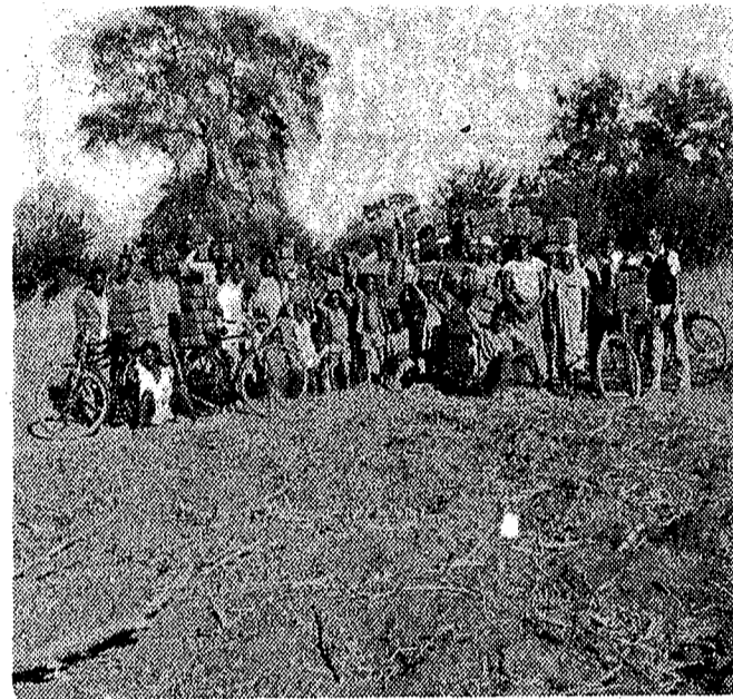
The church people transporting the bricks to the place where the new house will be erected; some people are carrying the bricks on their heads and some on their bicycles.
