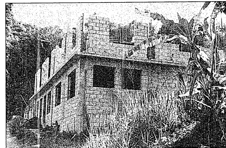
The walls begin to go up for the new Conference Centre at Maiden Hall, St. Mary, Jamaica.
