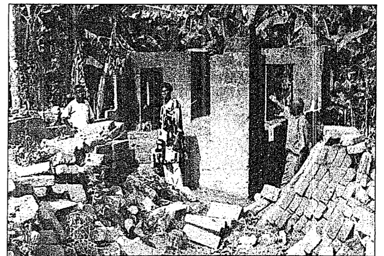
Pastor C.U. Marcus (right) surveys the damage to the SDB church following a recent storm in Nigeria.
