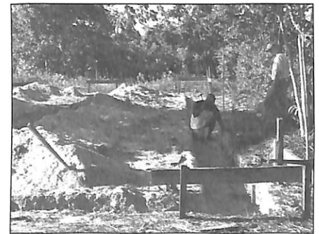
A hand-dug trench for the dorm's foundation greeted the American work crew.
