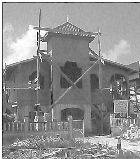
...during construction. The Guyana Conference now owns this building and the adjacent manse.
