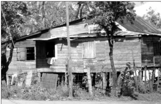
One of the homes damaged by Hurricane Felix.
