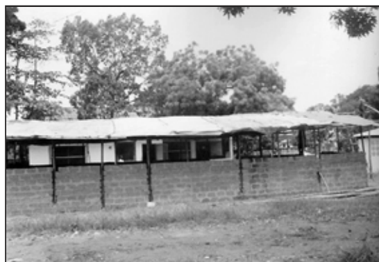
This unfinished school in Liberia needs better walls and roofing.
