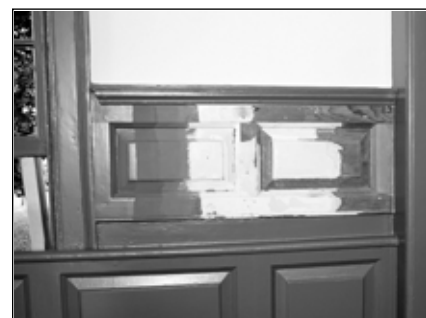
Example of the historical restoration, from bare wood at right to completion at left.
