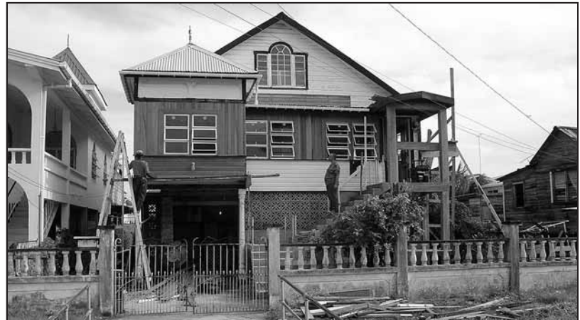
New windows and siding improved the exterior of the manse in Kitty, Guyana. The SDB church is at the left.
