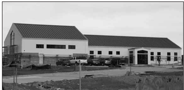
The Next Step Church in Thornton, Colo., as it neared the final stages of construction.
