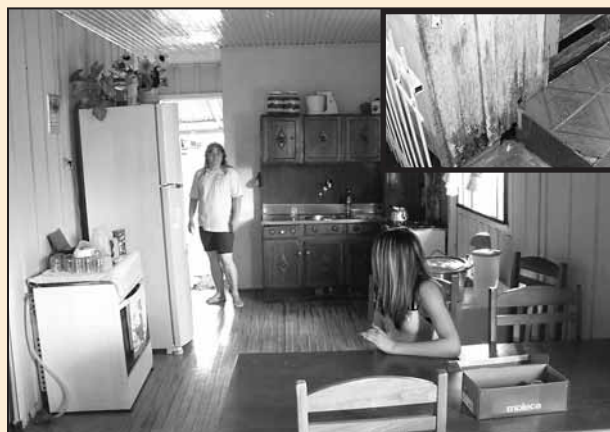
Notice the severe lean to the left, and the rotted wood outside (inset, upper right).
