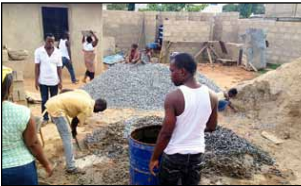
The Ghana SDB congregation has sacrificed time and funds to build a solid worship facility. Below: The interior nears completion.
